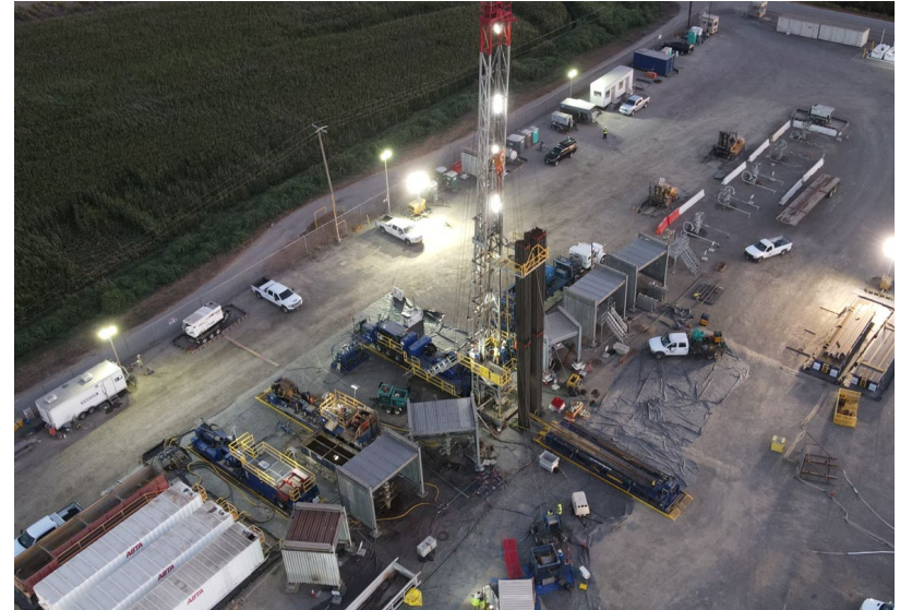
Typical well site with rig performing well inspection. Multiple wells are removed from service due to close spacing layout of facility.
