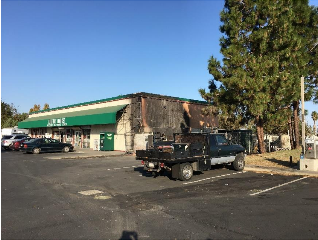
Figure 3: East side of the Gateway Gas & Mart suffered fire damage.
