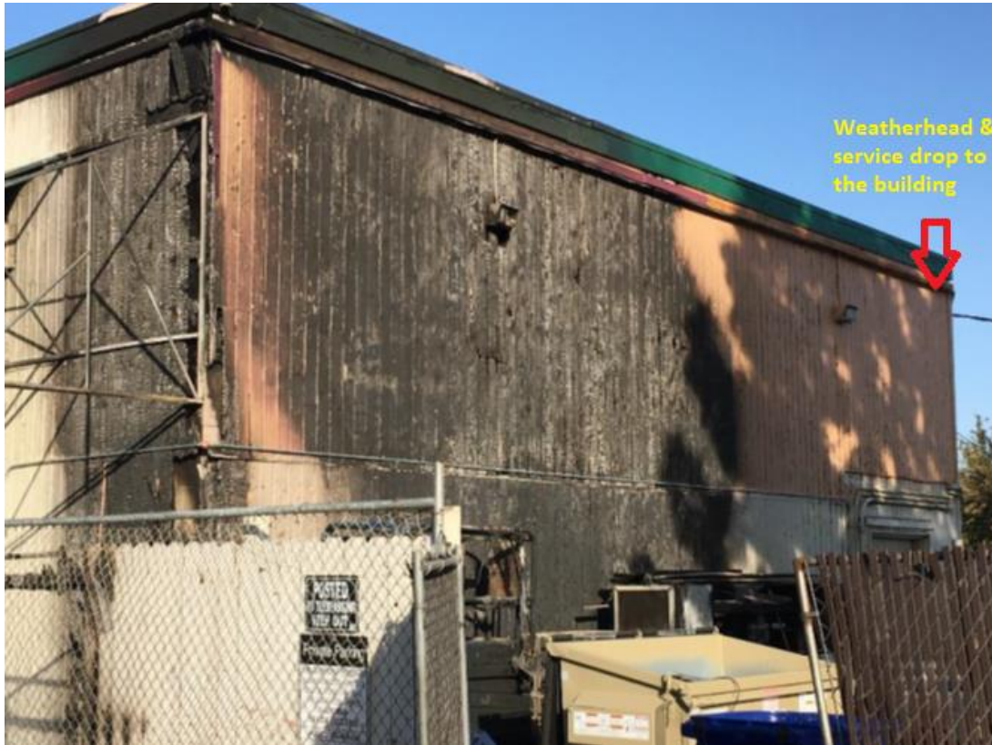
Figure 4: Closeup of damage at the Gateway Gas & Mart.
