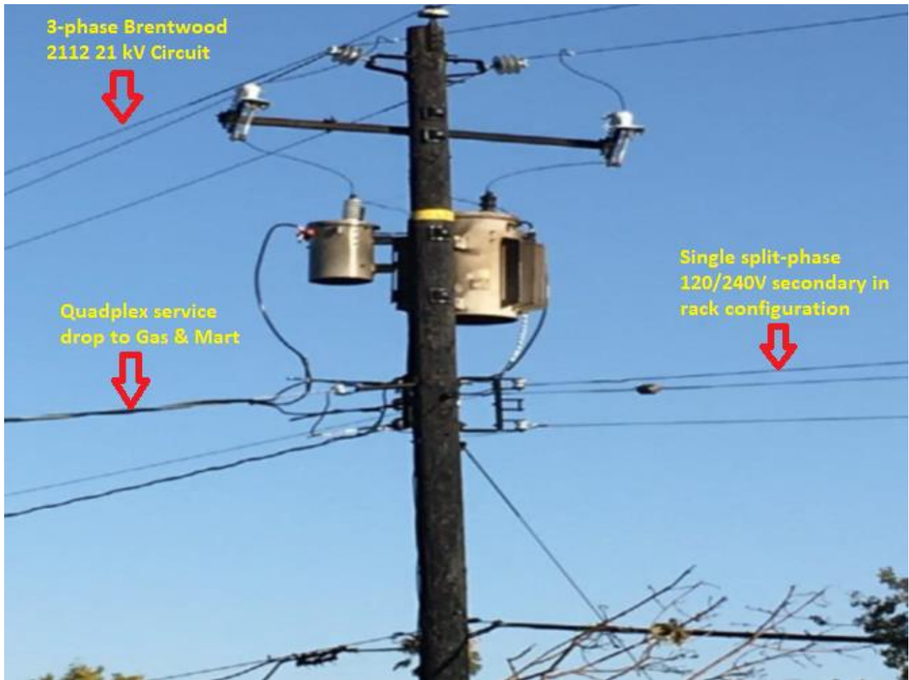
Figure 2: Pole #100457718 suffered char and burn damage from the fire. However, the two transformers were serviceable and put back into service after the fire.
