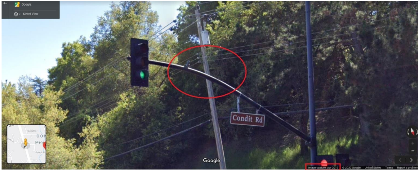
Figure 5. Google Street View image captured in April 2019 confirmed the communication cable had not yet been installed at the time. Source: Google Maps
