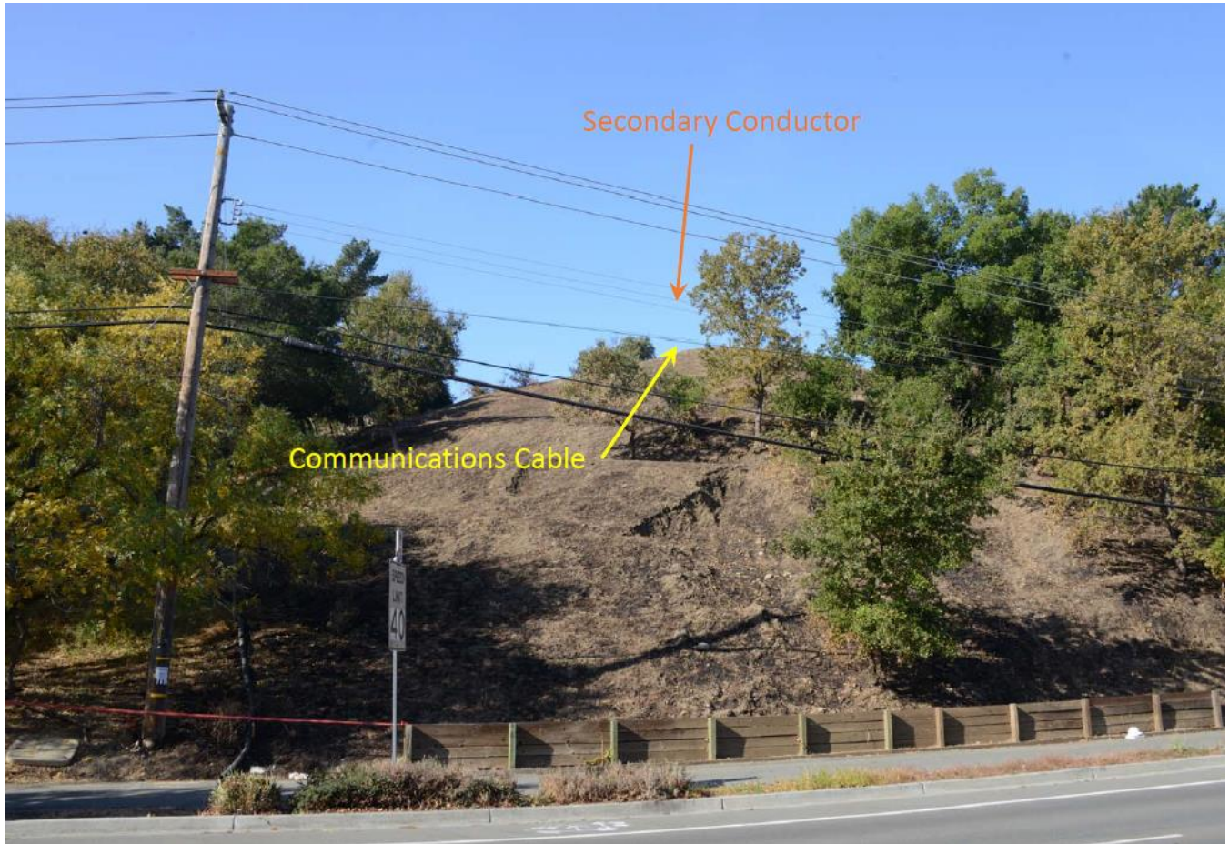
Figure 1. Incident location where the communication lash wire broke loose and contacted PG&E's Rossmoor 1104 12 kV secondary conductors.
