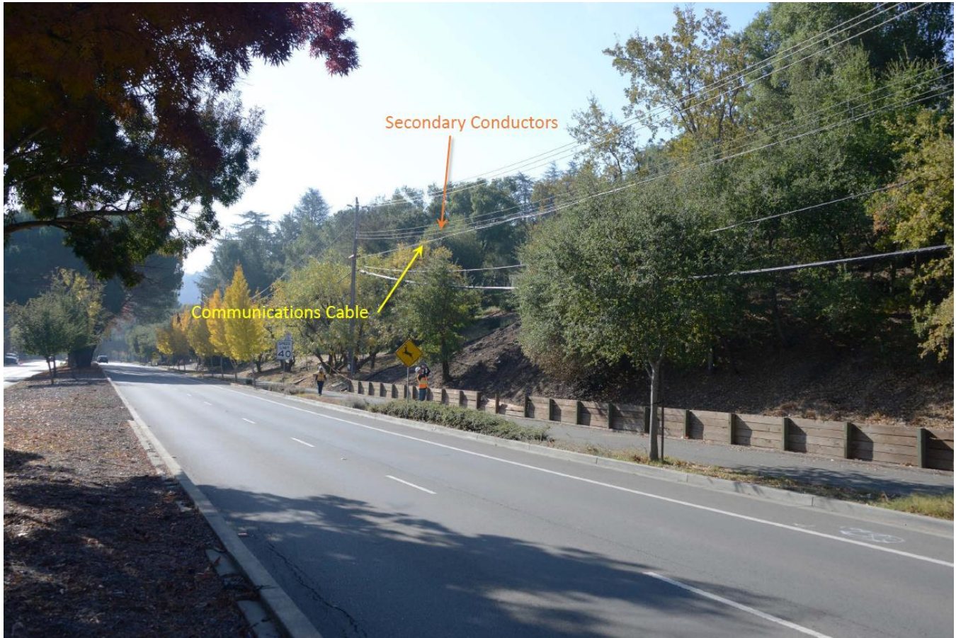
Figure 4. Photo showing the secondary conductors and communication cable are at the same height where the two made contact.
