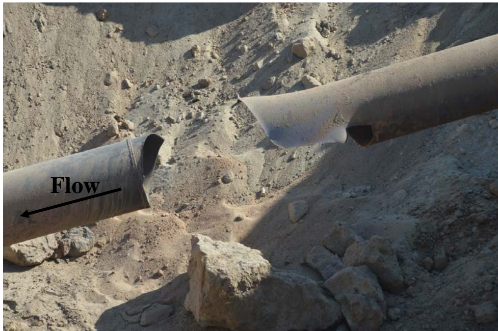
Figure 5. Photograph of the ruptured pipe segments looking northeast toward the dirt road and away from the railroad and Highway 99.
