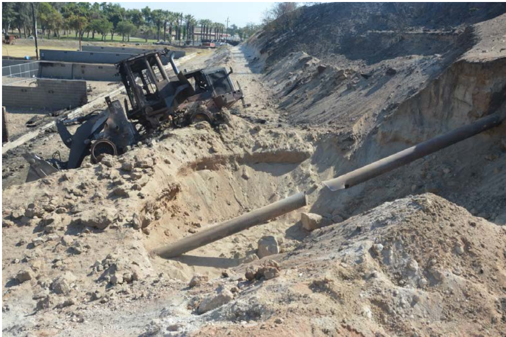
Figure 9. Photograph looking northeast at the ruptured pipeline and crater with the dirt road in the background. The uphill side of the road is coincident with the rupture location.
