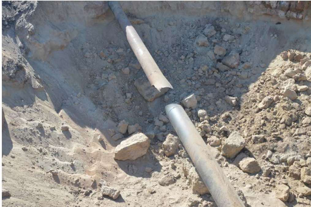
Figure 4. Photograph of the ruptured pipe segments taken looking upstream (southeast).
