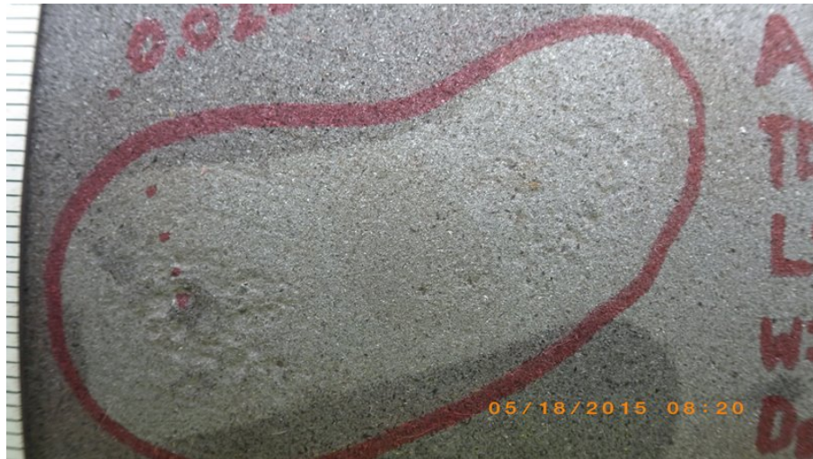
Figure 21. A representative example of minor external corrosion from Segment A (A-EC3).
