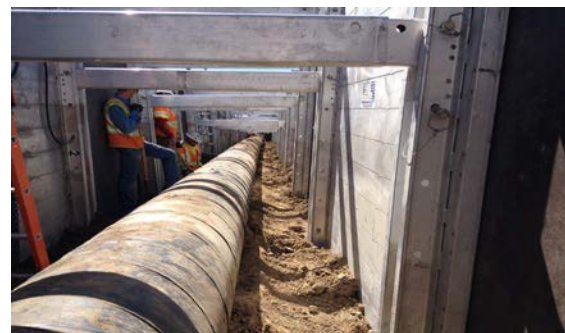
Figure 25 – Pipeline 21A As-found Condition After the 2014 Napa Earthquake
