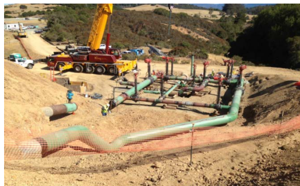
Figure 41 – Valve Automation at Edgewood Park
