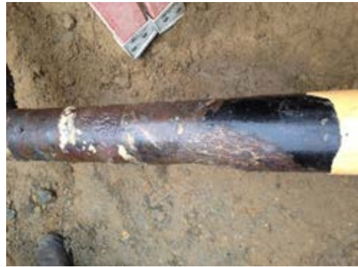
Figure 24 – Example of Corroded Pipe
