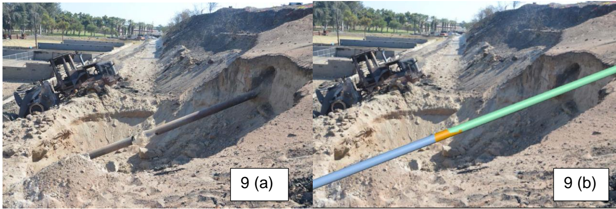
Figure 9: (A) Incident scene after the rupture, and (B) A Three-dimensional Reconstruction of the Pipe Overlaid on the Incident Scene
