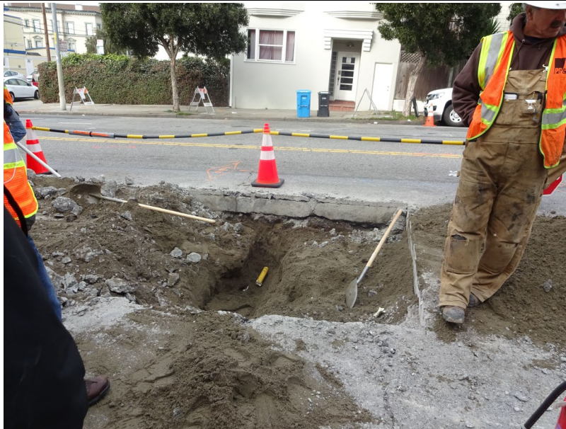
Figure 2. Photo of abandoned service tee location looking northwest towards [REDACTED]
