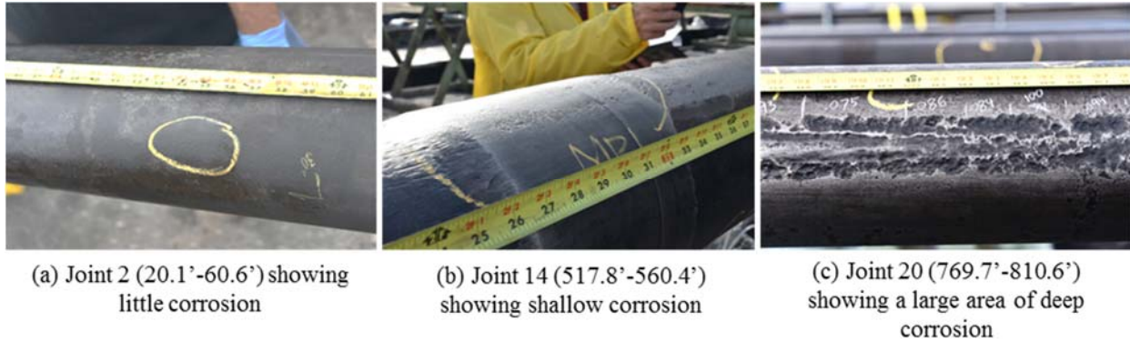
Figure 5: Severity of 7" casing external corrosion as a function of joint depth
