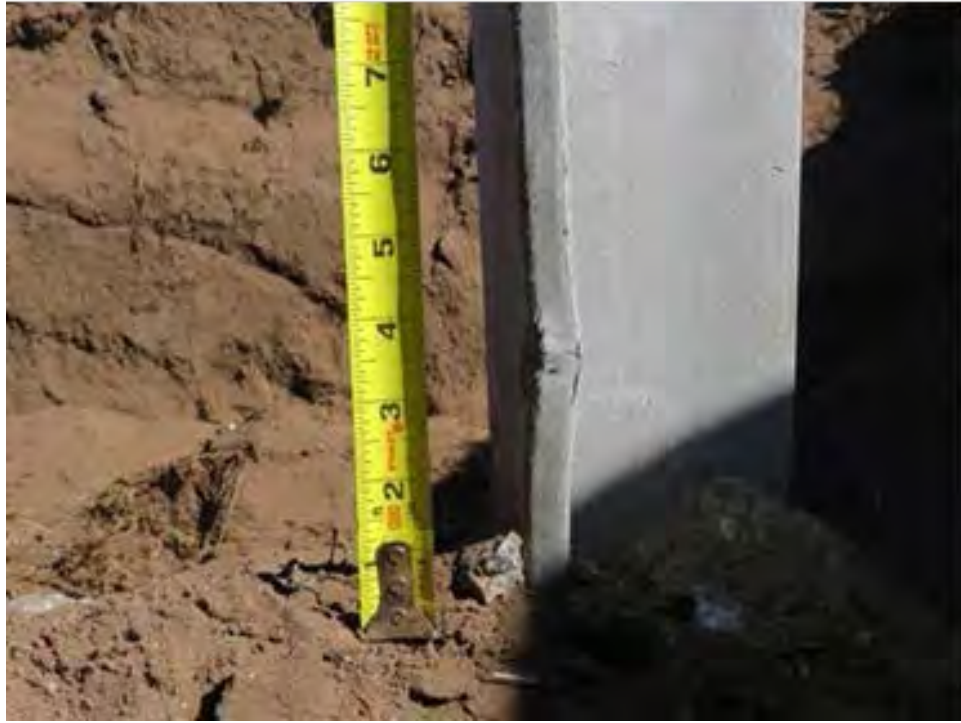
Figure 15. Deformation in Stub A
