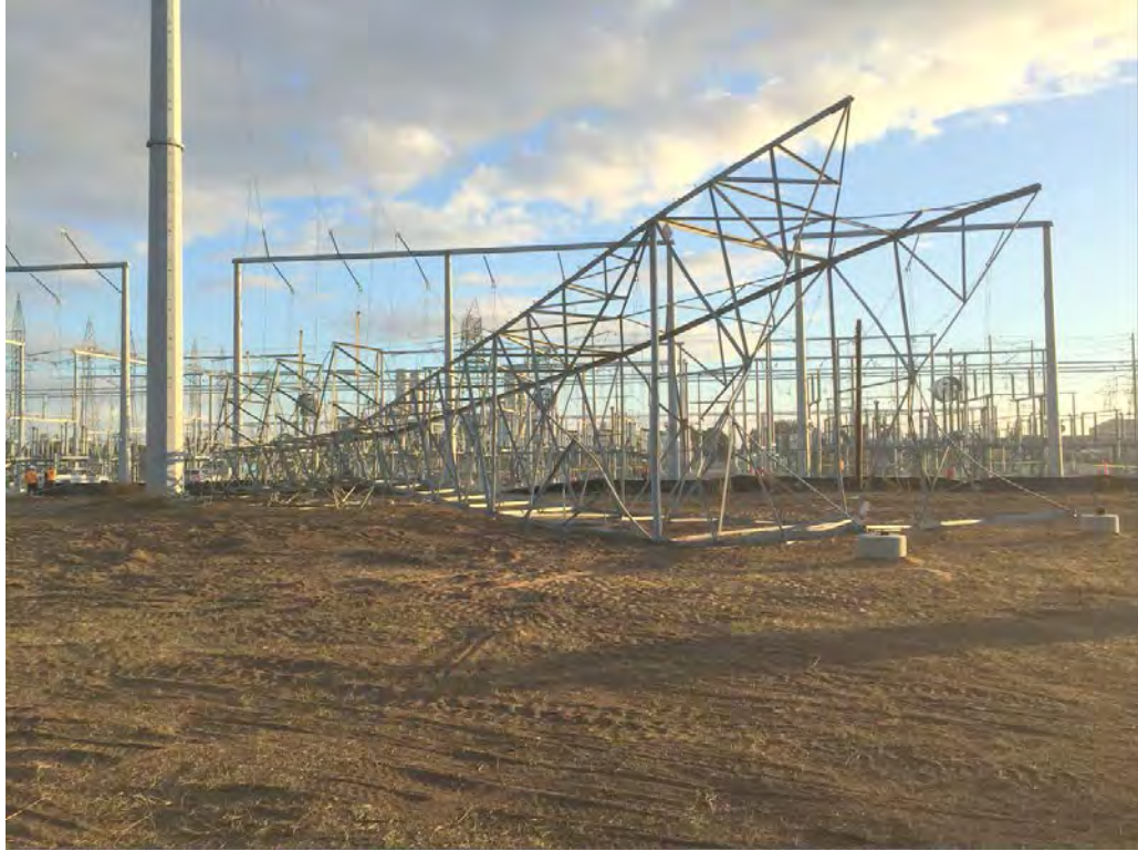
Figure 4. Failed tower as seen October 18, 2015. View to South.
