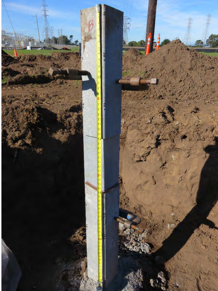
Figure 14. Measuring the plumb of stub angle on December 1, 2015 (extended to original height using additional angle sections)
