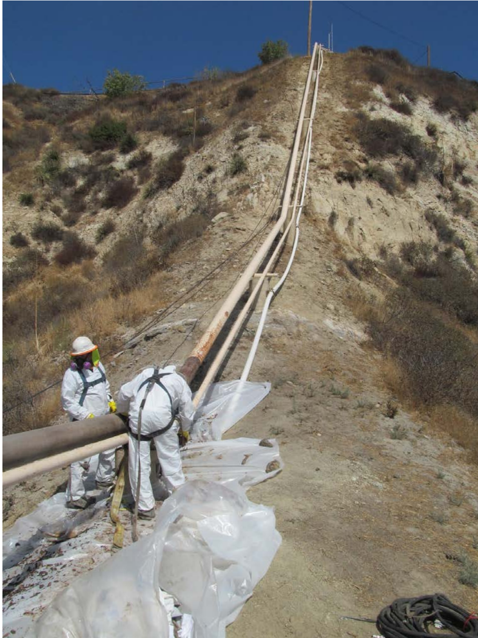
Figure 2. View from a location just upstream of the leak, looking east (upstream). Well location is beyond the top of the hill
