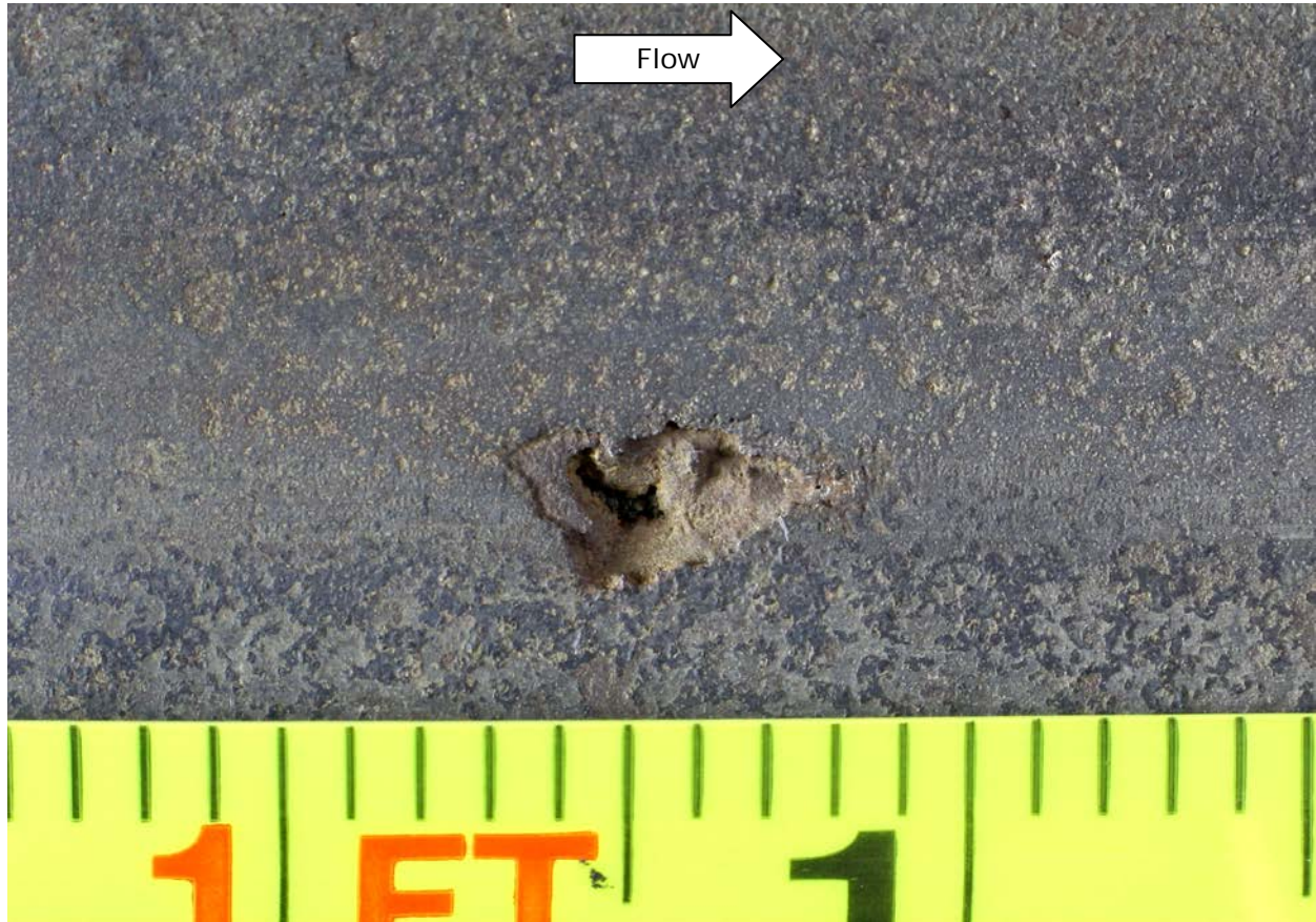
Figure 8. Photograph of the internal pipe surface at the leak/pit after cleaning.
