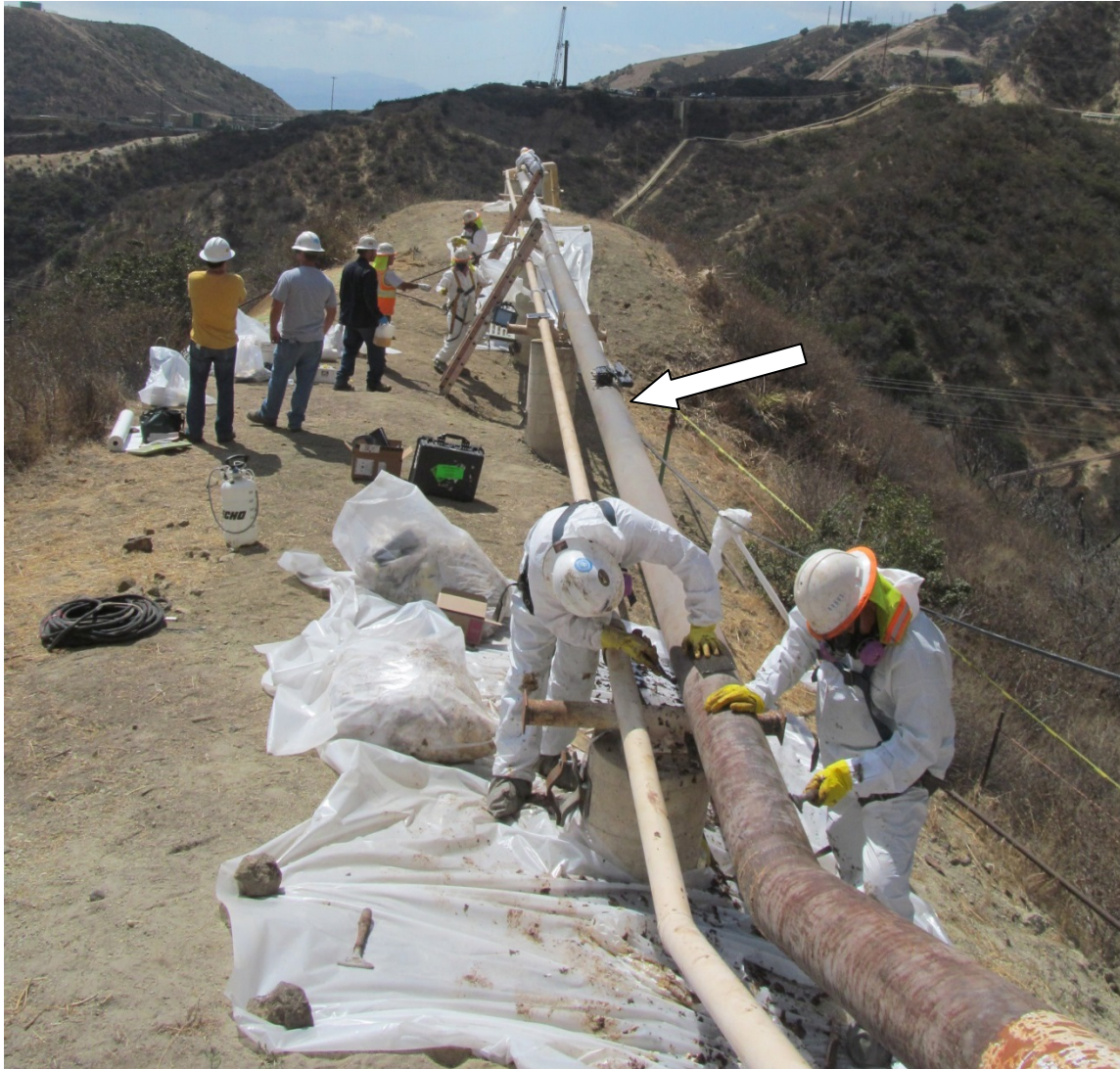
Figure 1. View of the well line looking west (downstream). Approximate axial location of the leak is indicated by the arrow. The pipeline is relatively horizontal here and the leak was at a slight sag or low spot.
