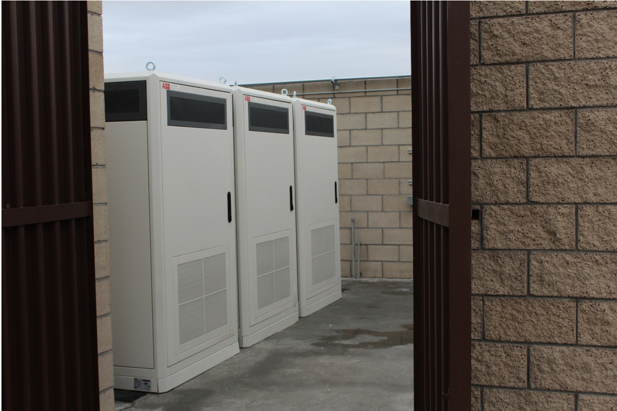
Figure 11 | ABB power cabinets. 1 cabinet feeds the 175 kW charger, 2 cabinets feed the 350 kW charger
