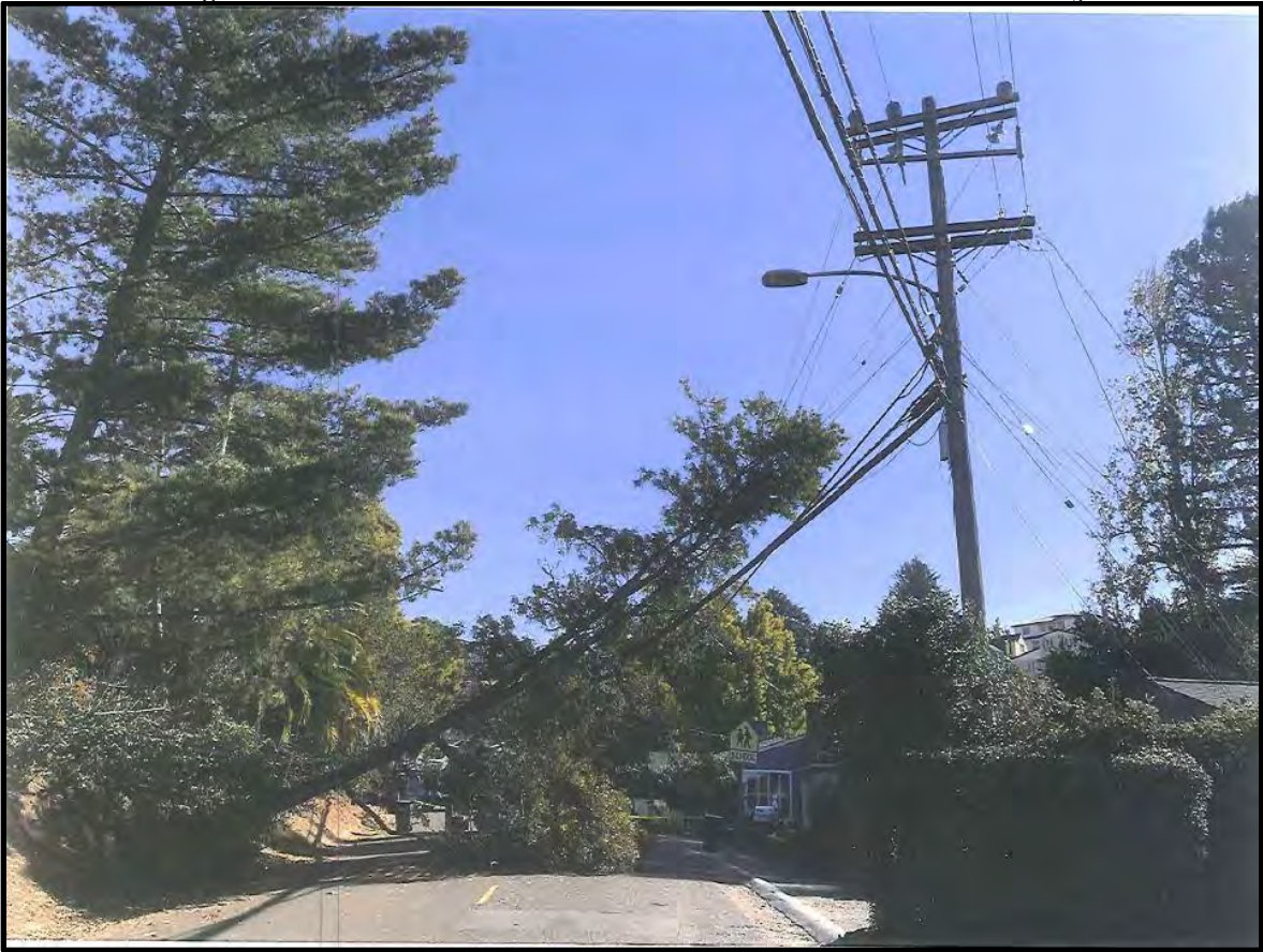
Figure 1: Tree fell onto conductors; Oakland, Alameda County
