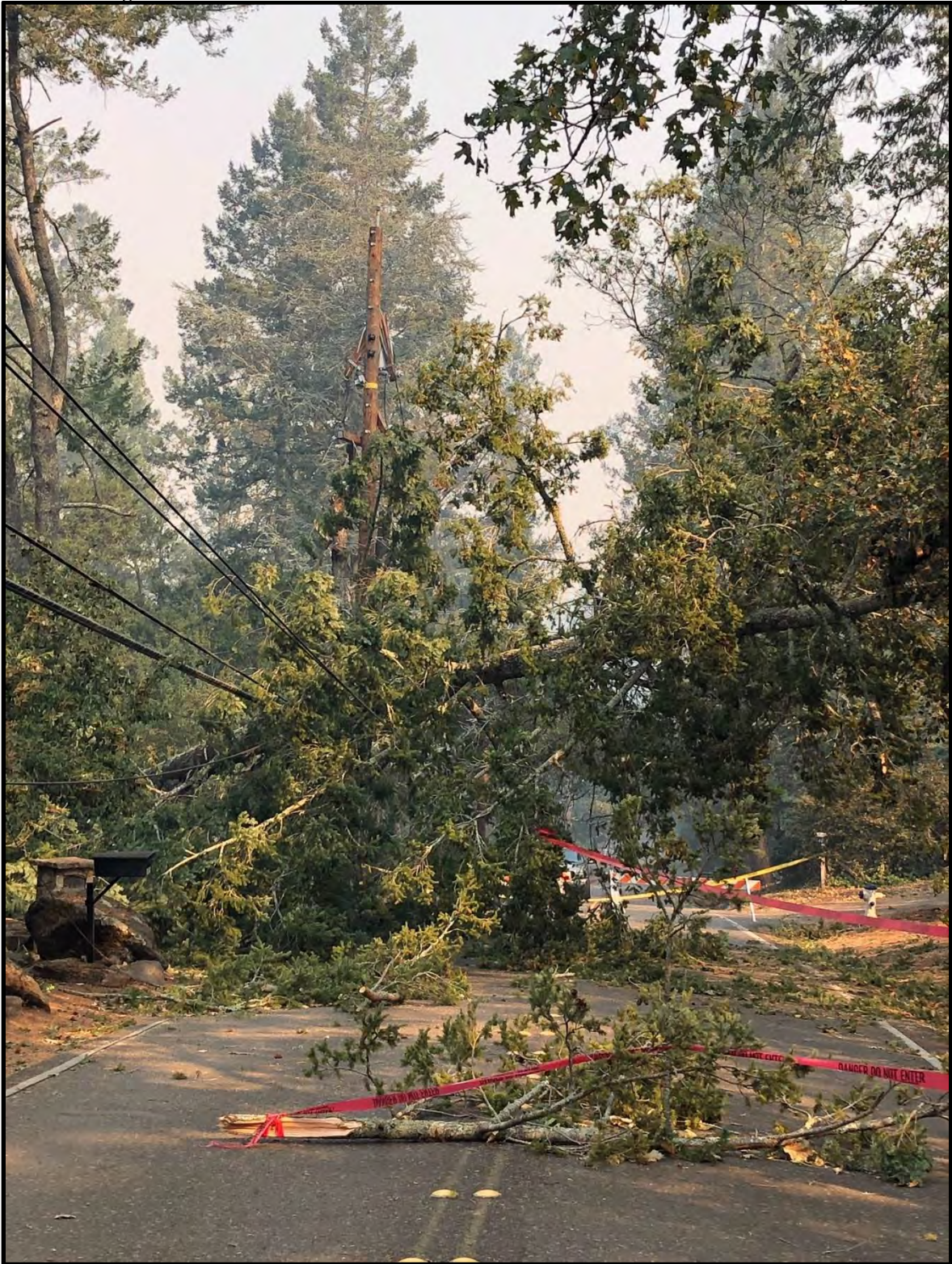
Figure 6: Tree fell, broken conductors; Santa Rosa, Sonoma County
