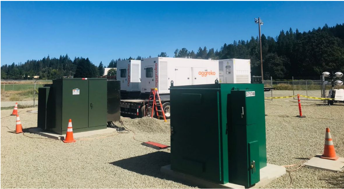
Figure 11: Mobile generation staged at Angwin's PIH on 9/23/2019
