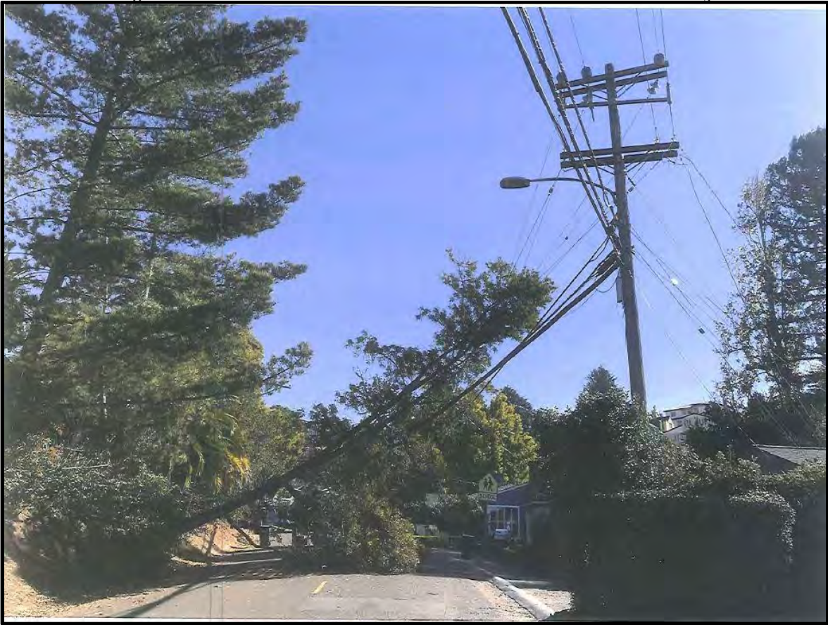
Figure 1: Tree fell onto conductors; Oakland, Alameda County
