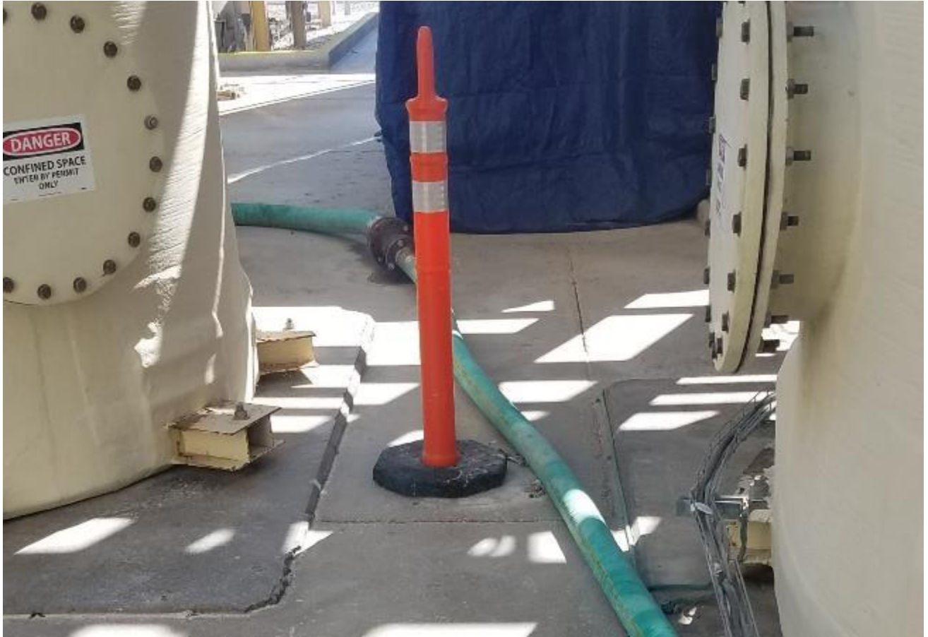
A hose in the walkway at the Beta Plant.
