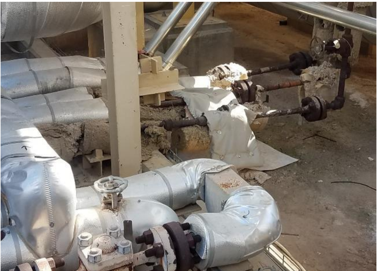
An example of damaged insulation at the Beta Plant.
