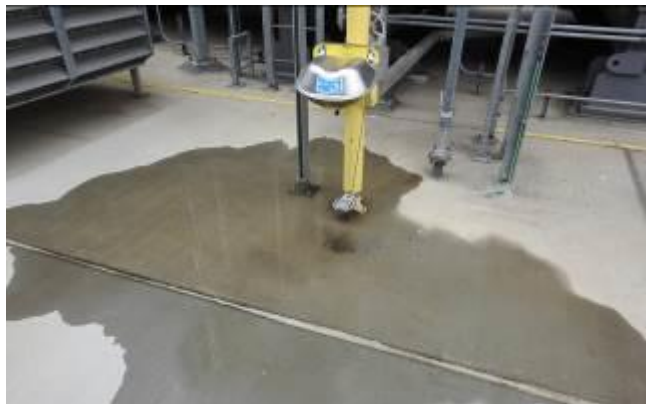
Leak from the shower station by unit 9 and standing water.
