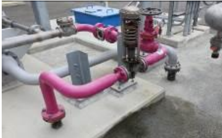
Leak from a valve on the evaporative cooling piping for unit 10
