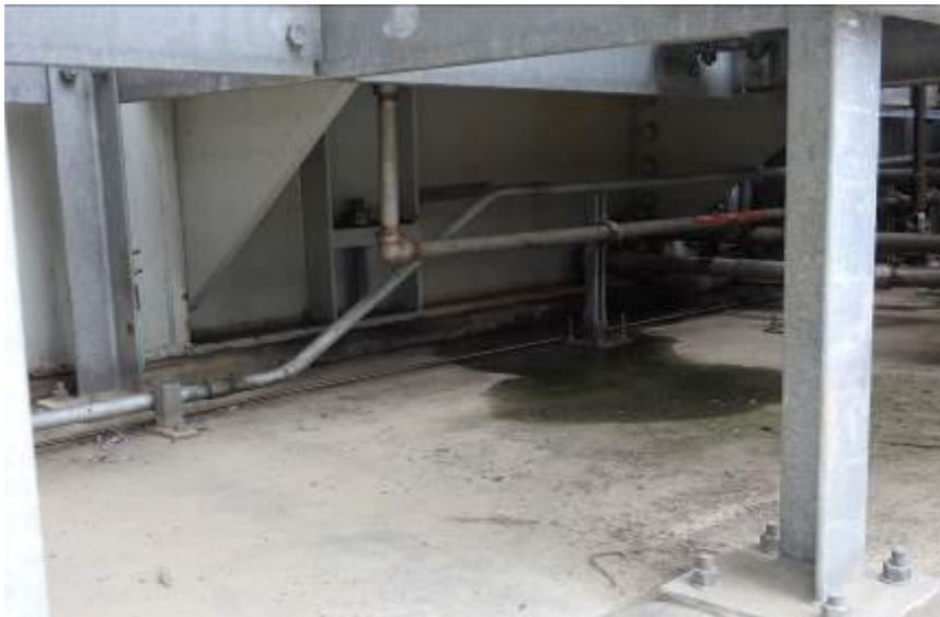
Evidence of a leak and standing water under the turbine compartment of unit 9.
