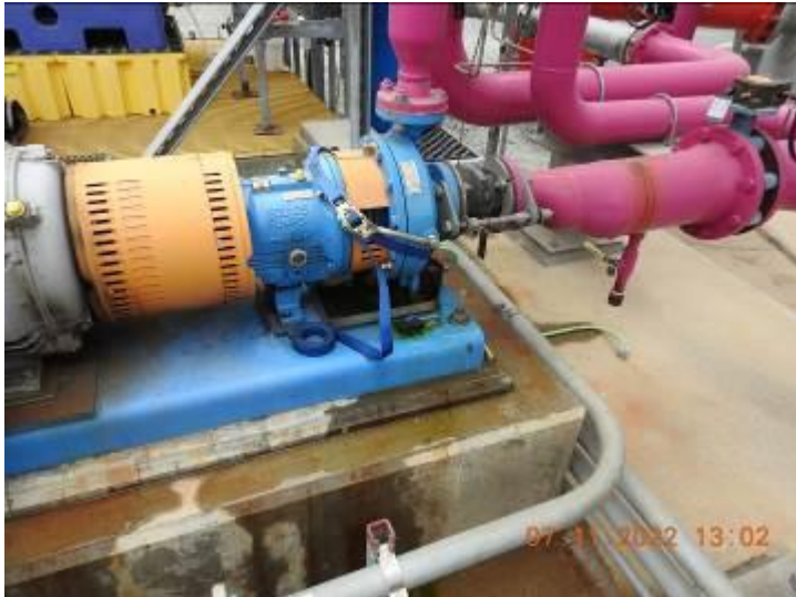
Leak from a reclaimed water pump near the reclaimed water tank.
