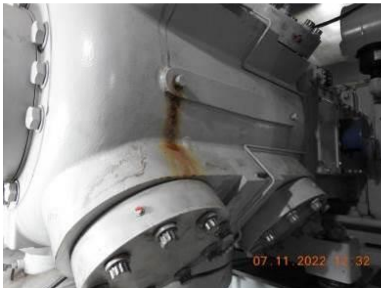
Evidence of a leak from a bolt on the gas compressor on Compressor A.
