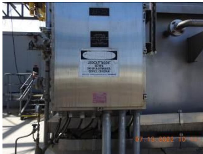
Faded danger sign on unit 7 near the turbine compartment
