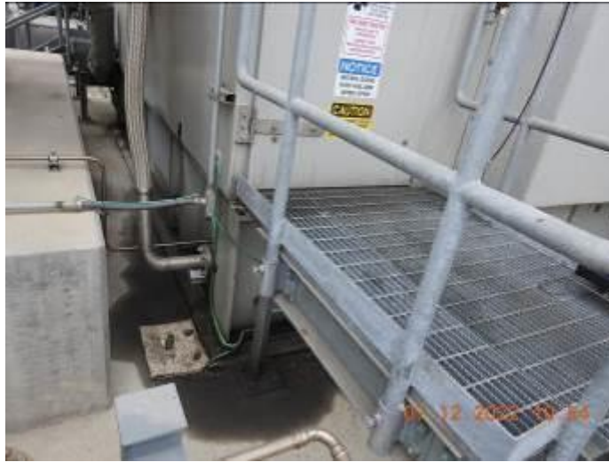
Evidence of a leak under the power turbine/generator compartment on unit 8.
