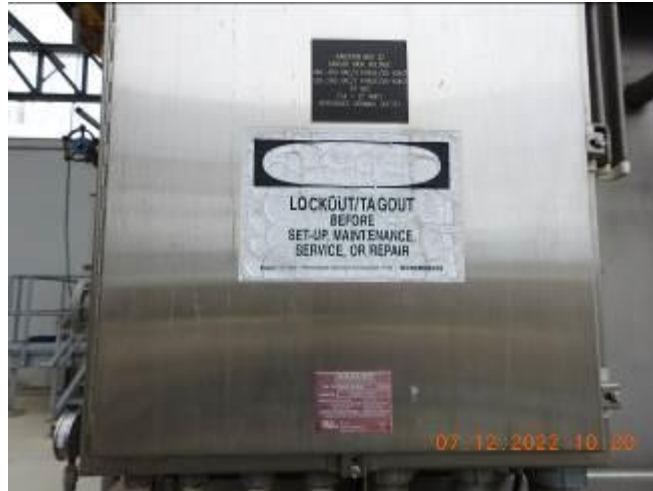
Faded danger sign on unit 9 near the turbine compartment
