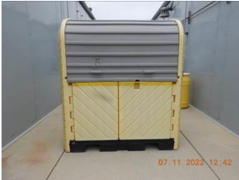
Used oil storage without an NFPA sign (fire diamond)
