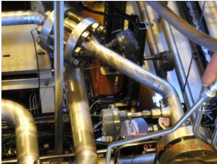
Standing water in the turbine compartment on unit 6
