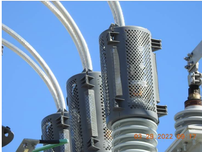
Bird protection cages covering oil sight glass on transformer bushings.
