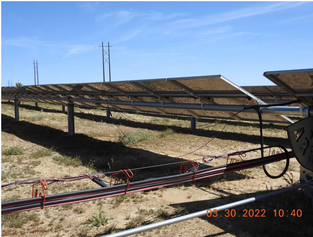
Cables detached from panels close to ground.
