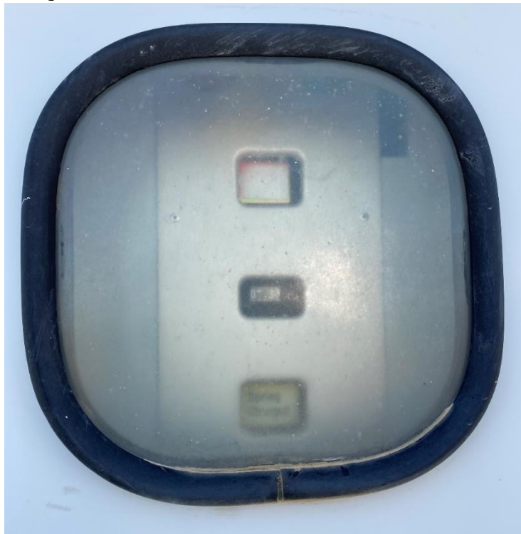
Figure 7: Illegible counter (middle) and faded breaker position indicator (top).
