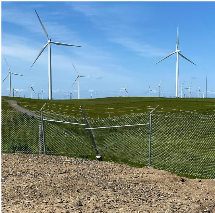
Figure 2 : Damaged and washed out fencing [REDACTED]
