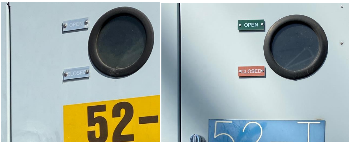
Figure 3: Faded “OPEN” and “CLOSED breaker labels (left), compared to another breaker’s labels in the Montezuma I substation (right).
