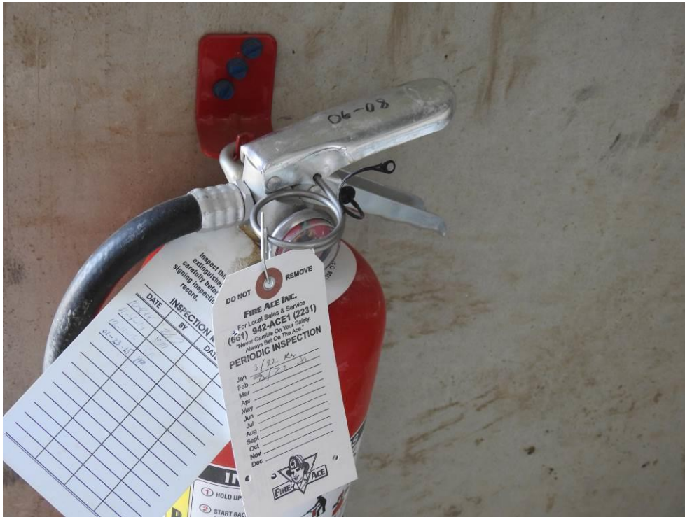
Tamper Seal not properly installed on Fire Extinguisher
