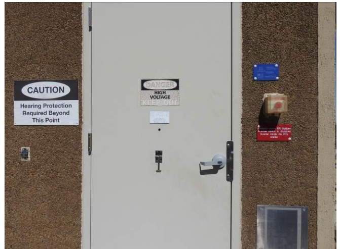
Faded High Voltage sign
