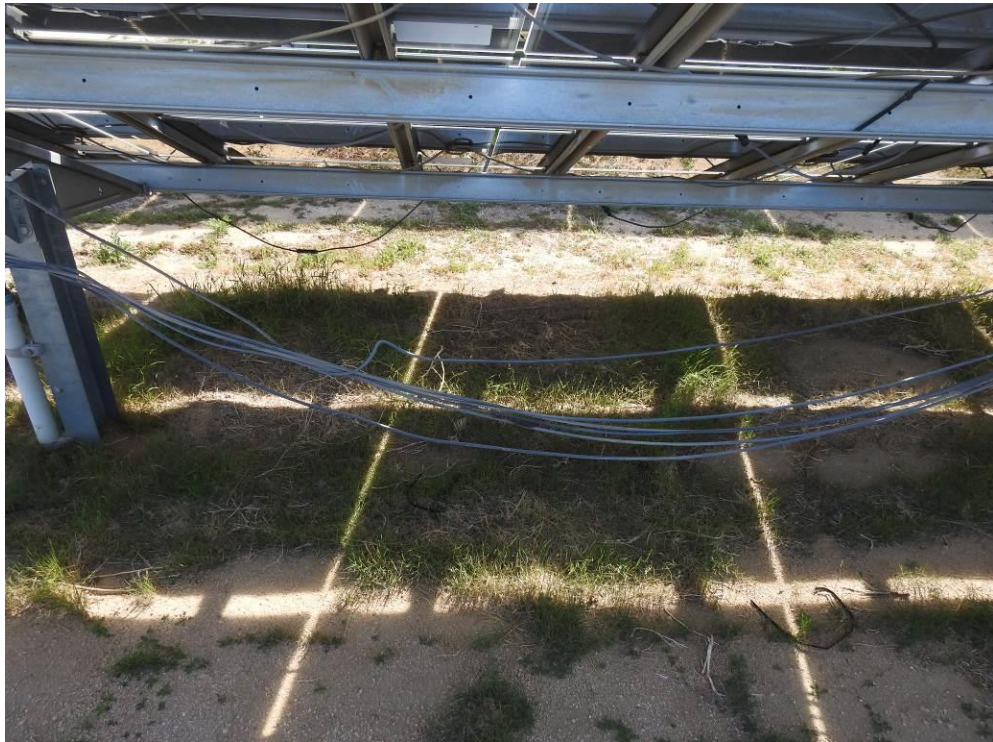
Cables detached from panels close to ground.
