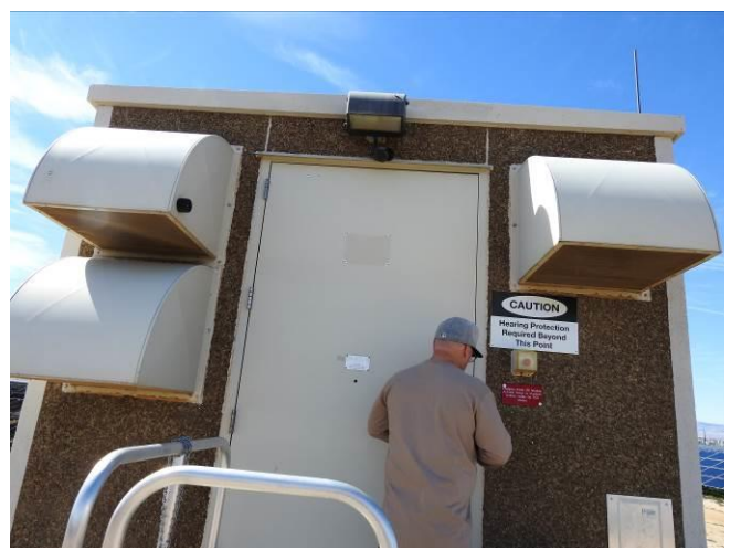
Missing High Voltage sign
