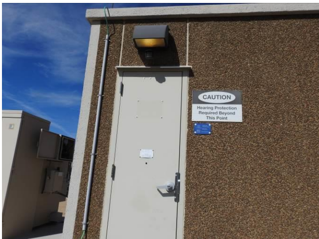
Missing High Voltage sign
