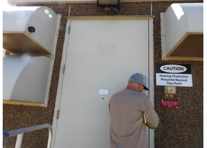
Missing High Voltage sign
