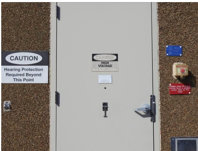
Faded High Voltage sign
