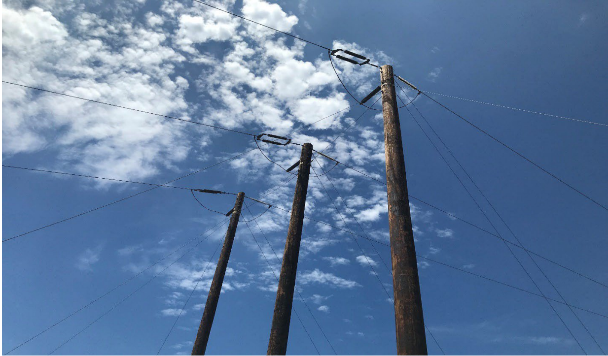
Figure 4. Photo of the configuration of the three Incident Poles (looking in the southwesterly direction toward Moro Ridge Road).
