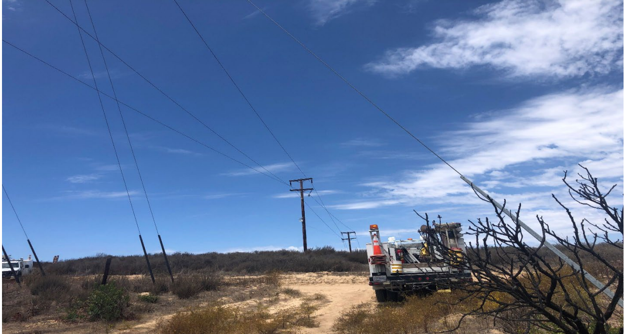
Figure 7. Photo of a single pole supporting three conductors west of Moro Ridge Road.
