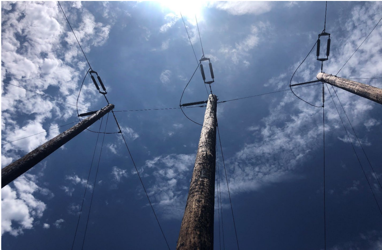
Figure 10. Photo showing the conductor and equipment supported on Incident Poles.
