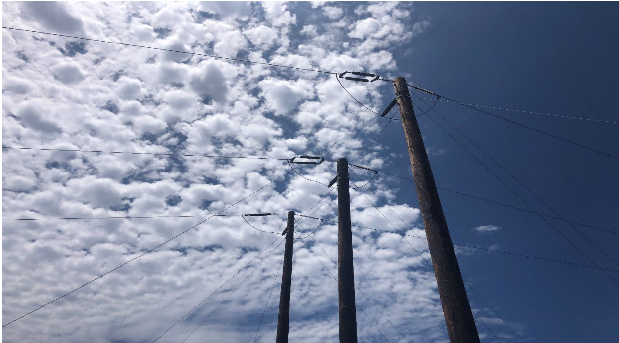
Figure 8. Photo of the Incident Poles showing conductor, equipment, and guy wire support.
