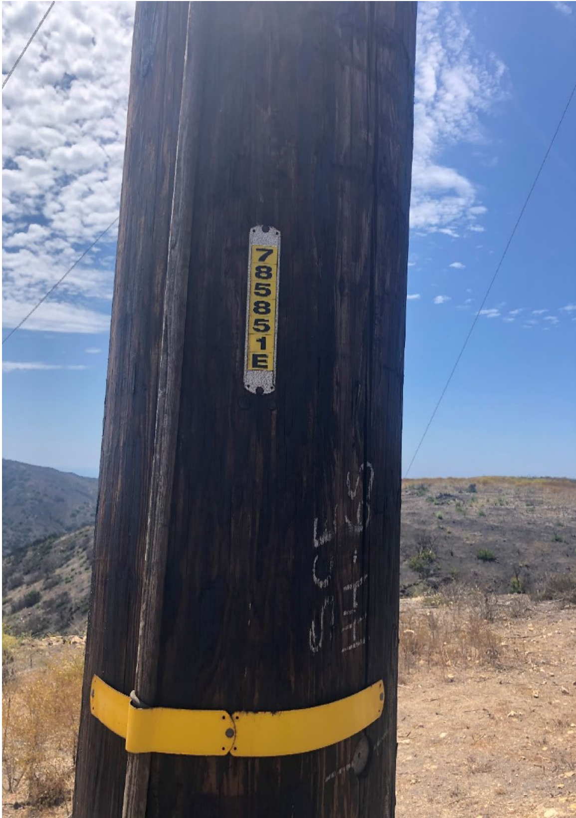
Figure 9. Close-up photo showing the condition of one of the Incident Poles supporting one of the conductors.
