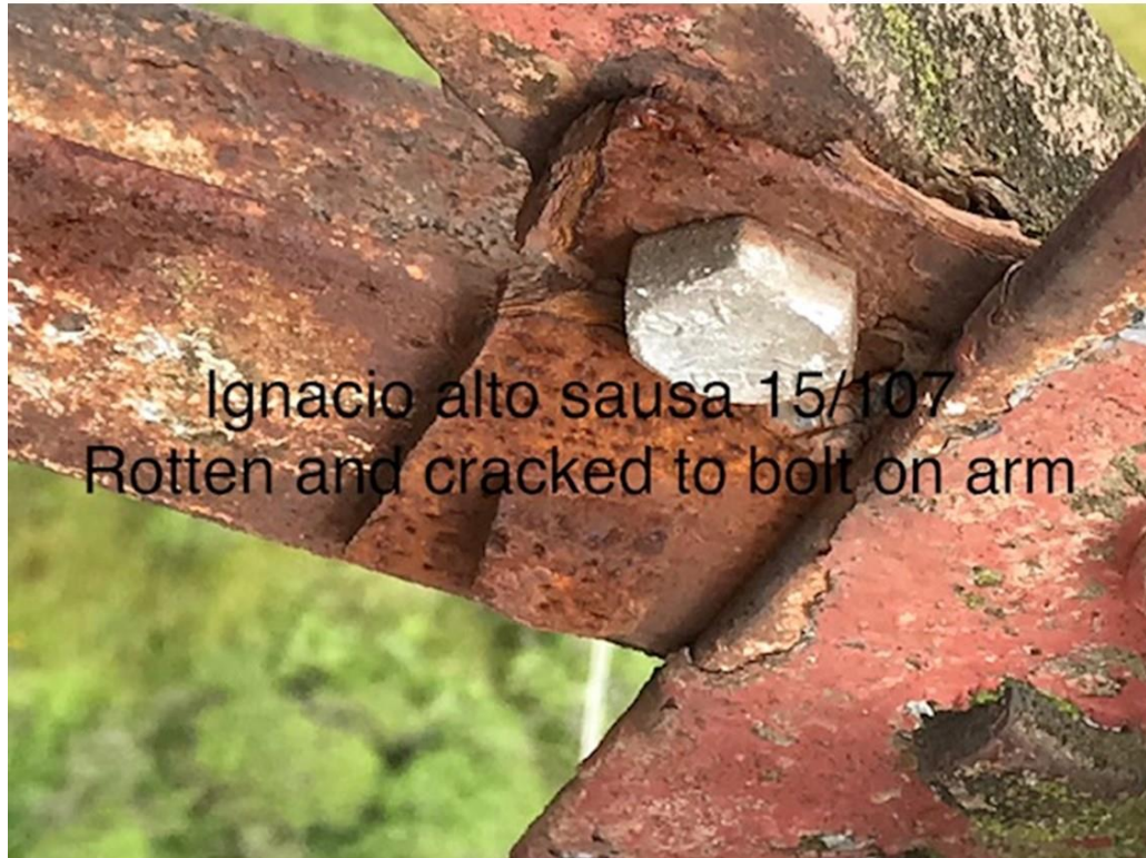
Figure 2: Identified Deficiencies on Tower # 15/107
