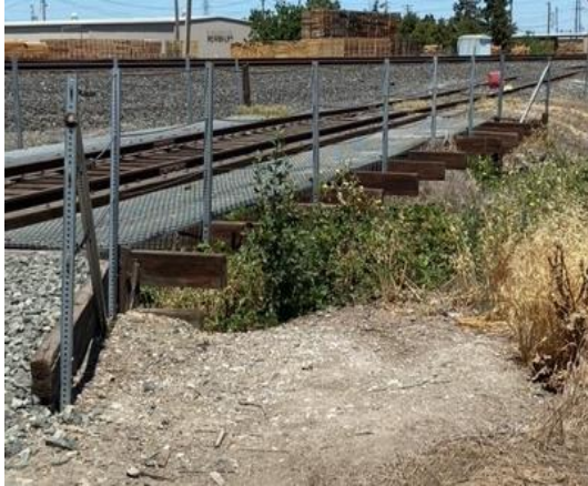
Before: Vegetation growing around the bridge
