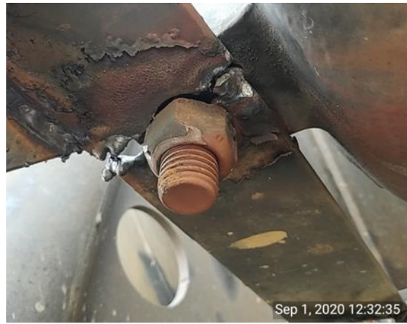
RSD Mechanical inspector discovered the air reservoir tank mounting brackets were broken and not properly repaired. The train brakes on this rail car may become ineffective due to this defective condition.
