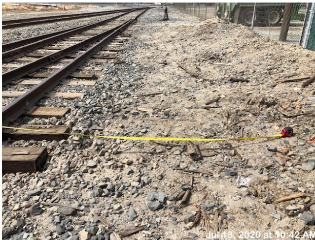
Before: Irregular walkway surface
