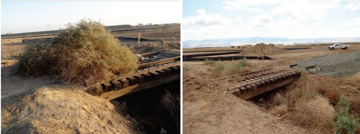
All American crude oil terminal in Bakersfield. The January, 14, 2014 photo, left, shows preliminary site stakes in the ground just to the right of the overgrown bush. Within just three months, the March, 27, 2014, photo, right, shows train tracks placed – quickly constructed to make the facility ready for receiving crude oil transported by rail.
