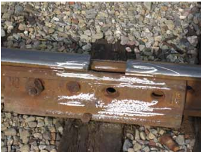
Close up view of track separation on inside of track
