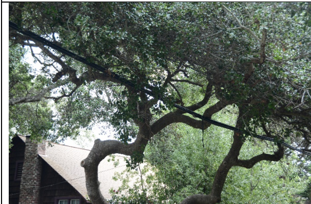
Cables rubbing against tree branches
