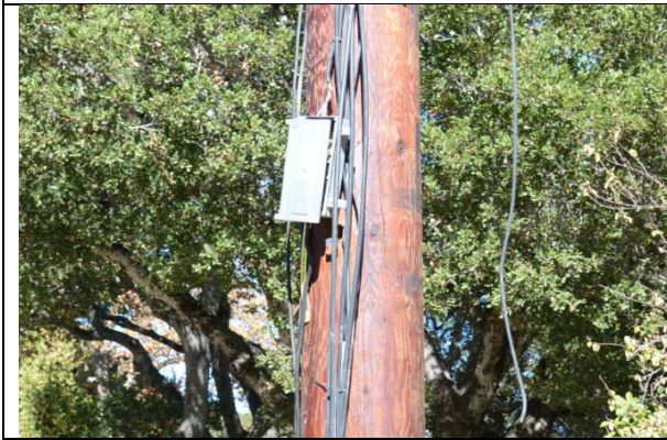
Terminal and drops
