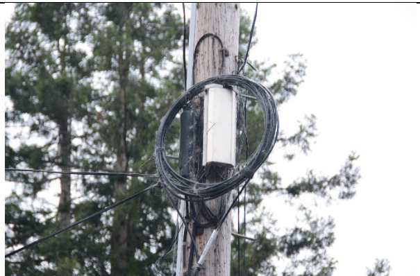
Deferred maintenance (San Geronimo)
