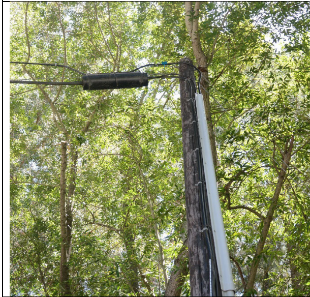
Unprotected cables on riser pole
