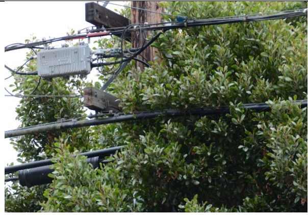
Overgrowth of trees near facilities
