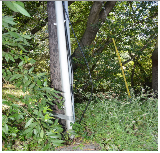
Cables detached and unprotected
