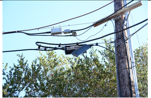
Terminal improperly attached
